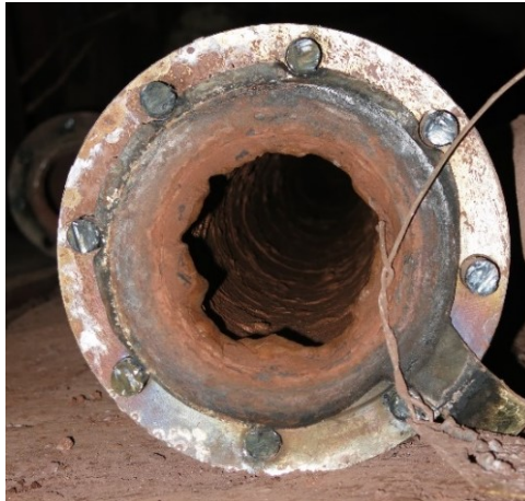
Figure 6. Slurry scale in pipe from sump pump.
